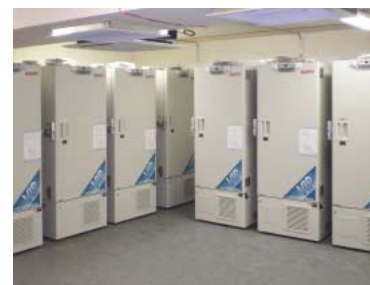
A view of some of the twenty MDF-U53V Freezers installed in the new Biorepository at the University of Sheffield.
